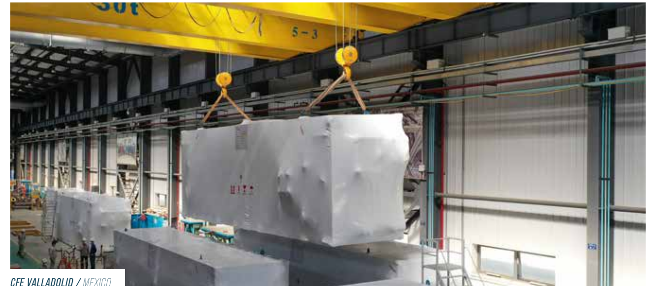
CFE VALLADOLID / MEXICO
